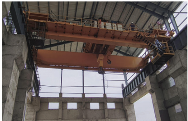
POWER HOUSE-I (VIEW FROM SERVICE BAY)
