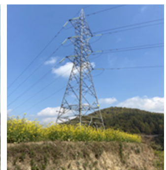
Visit to the proposed 220/132/33kV substation site at NalaGumba in Kathmandu Valley
