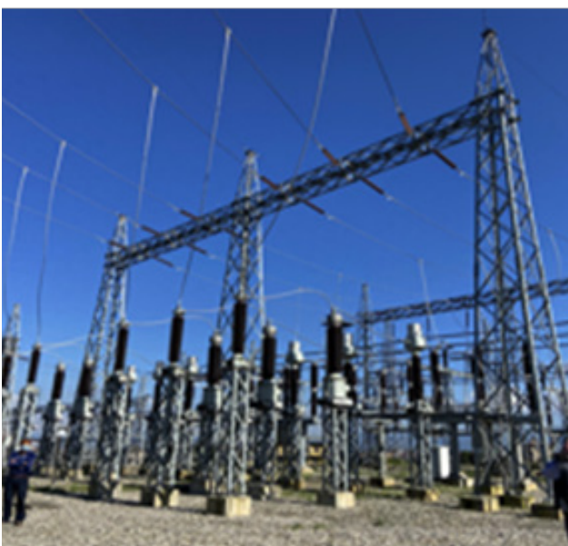
Visit to 220/132/33/11kV Matatirtha substation in Kathmandu Valley
