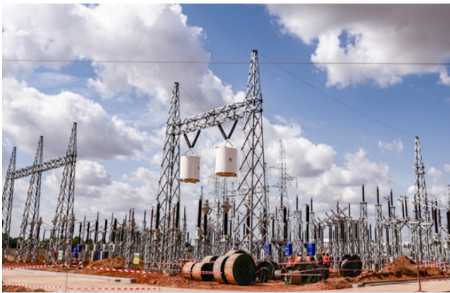
Switch yard view of Dapaong substation
