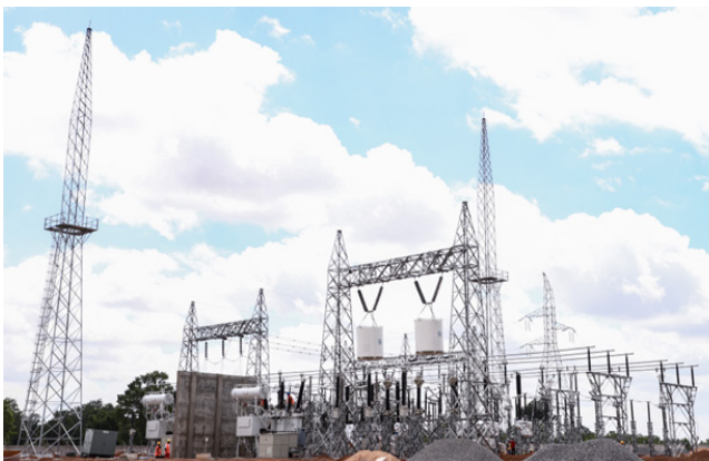
Switch yard view of Mango Substation
