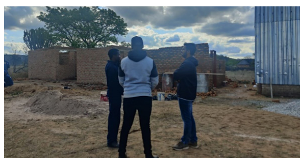
Visit of WAPCOS team for one of the sites as a part of Construction Supervision
