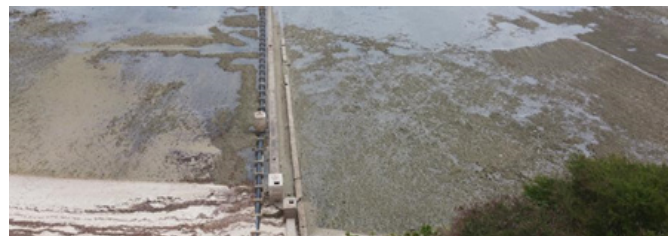
Discharge Pipe into the Sea at Raskazone (Jet Sea Outfall)
