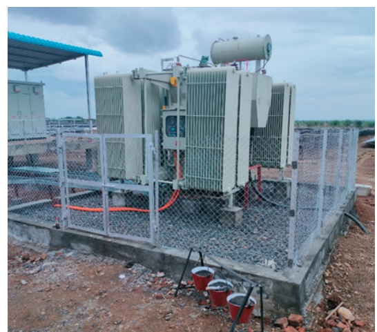
Installed Inverter Duty Transformer (IDT) of 5 MVA Capacity
