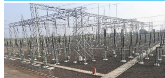
Pooling Switchyard 33/220 KV
