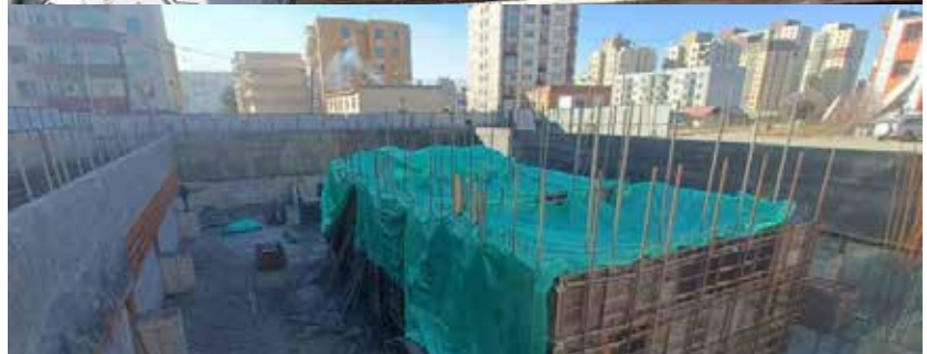
Main Building Sub Structure above the Raft Foundation upto (+) 0.85 Lvl including Retaining wall Pedestals (-)3.75 Lvl, Water Tanks upto (-) 0.85 Lvl, Service Lift and Passenger Lifts
