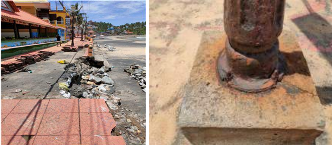
Figure 4-8 Damaged pedestrian pathway (left); Damaged Lamp Post (Right)
