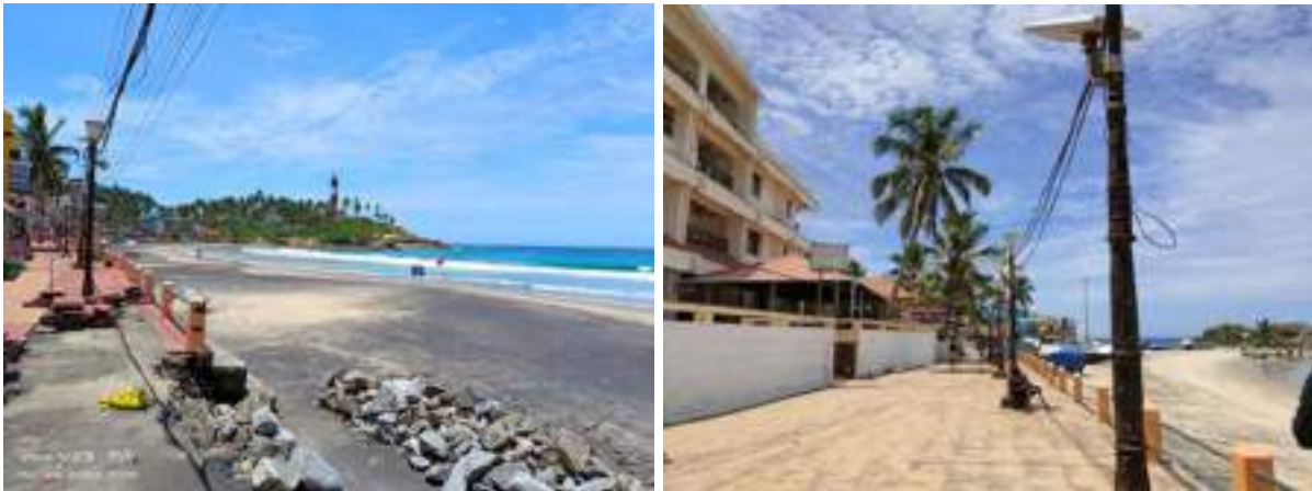
Figure 4-1 Dilapidated Condition of the Pathway at Light House Beach (left); Overhead Lines and Light Posts at Light House Beach (Right)
